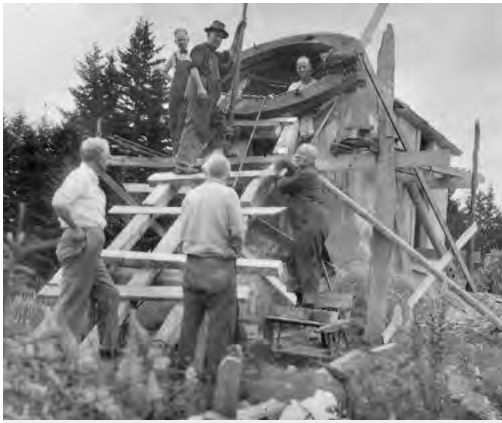
Jacking the heavy RA ring into position during the Porter Turret's construction. The telescope could only have been built in a place like Springfield, where the Jones & Lamson Machine Company, employer of Porter and others, afforded members the means to machine large parts.
